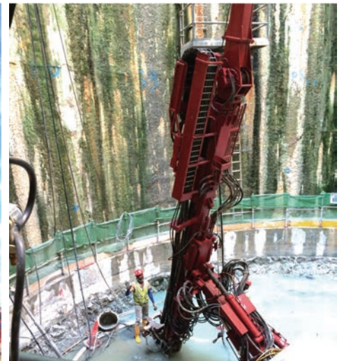
Transnission Cable Tunnel NS2
